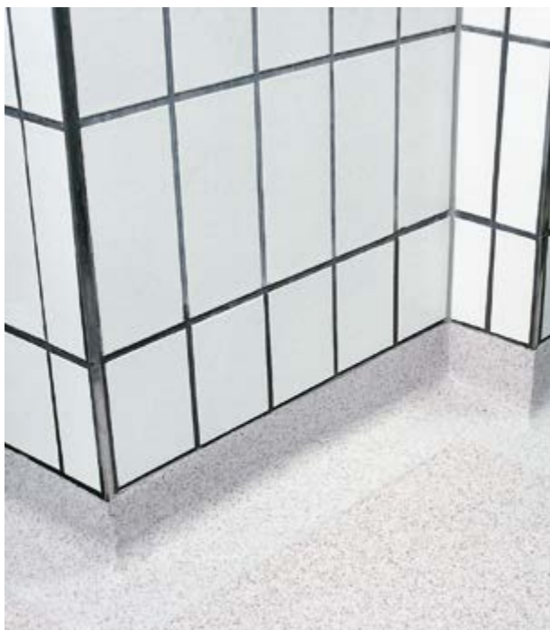
Coving in the composite are worked into a smooth surface on the tiles.
