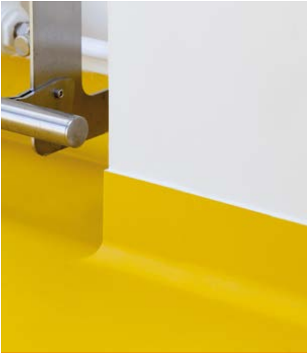
Covings are implemented by hand on the walls of a pharmaceutical cleanroom or operating room.
