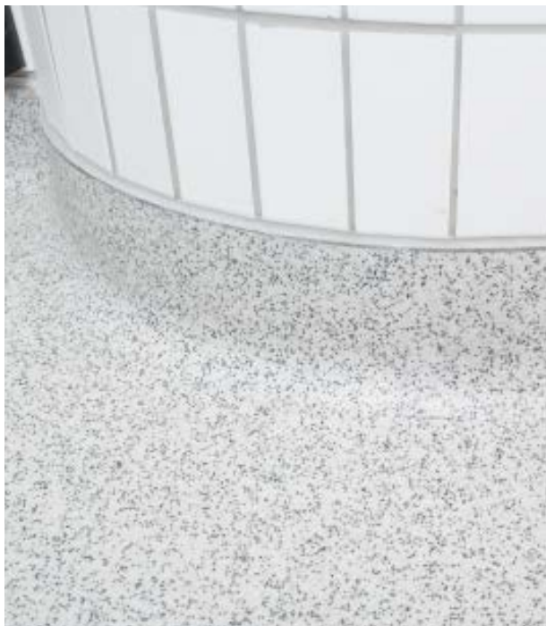
Coving for the composite are modeled into a smooth surface on the pillars.
